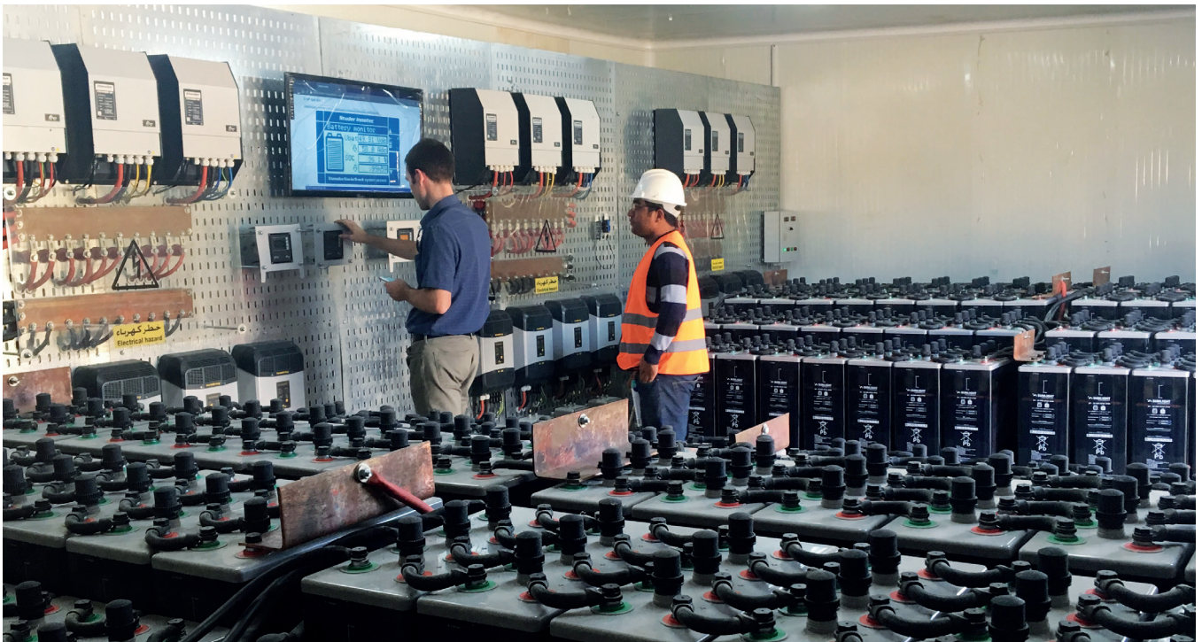
Centralised solar street lighting installation, Egypt. Photo credit: Hammer Electric S.A.E.
