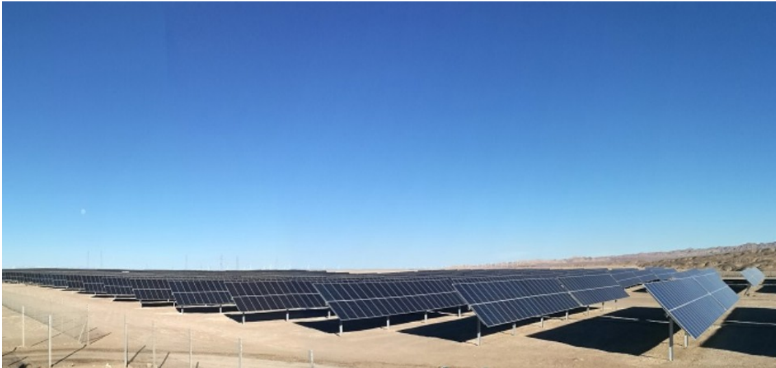
Photo: Puerto Seco Solar Park, Antofagasta region, Chile
