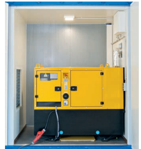
Generator in an autonomous container
