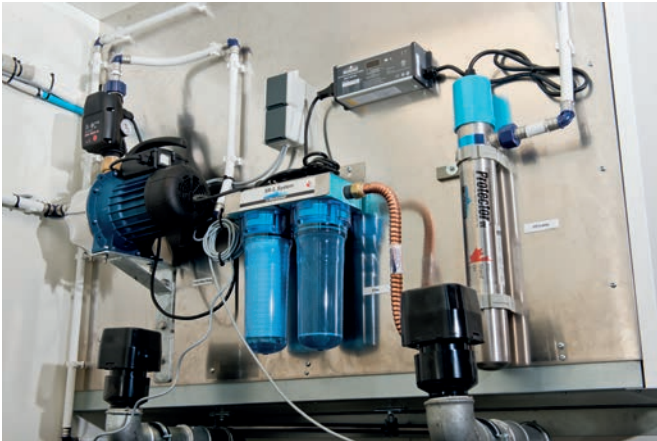
Filter system and UV lamp in an autonomous container
